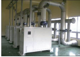
WWTP of Hoeya, Ulsan (NX150), Korea
