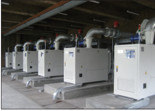
WWTP of Daejeon(NX200), Korea
